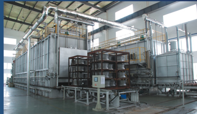
T4 & T6 Heat Treatment System
